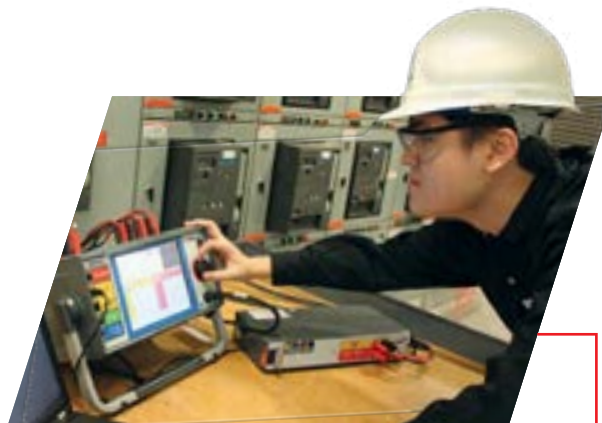
Protection relays and systems
